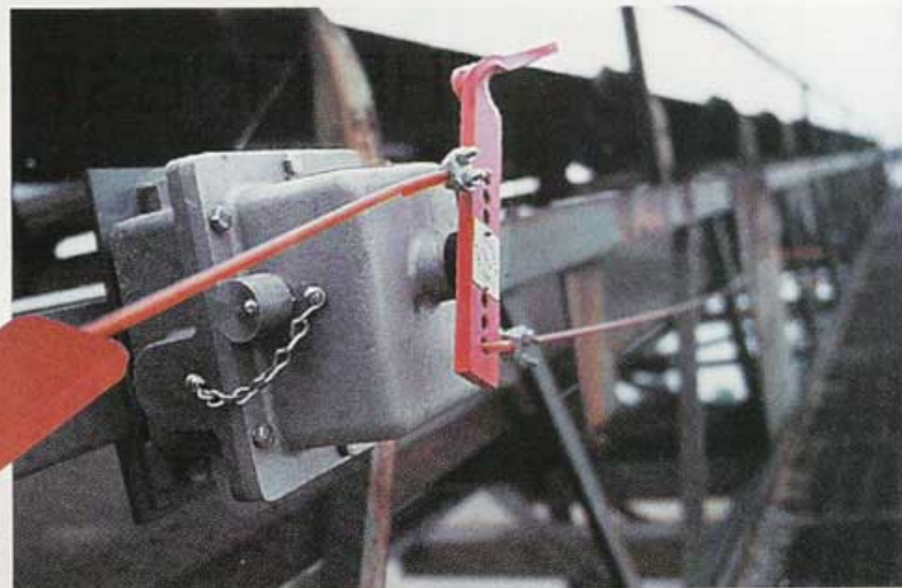
The model RS Safety Stop Switch in operation for immediate shutdown of conveyor system at a sand and gravel company.
